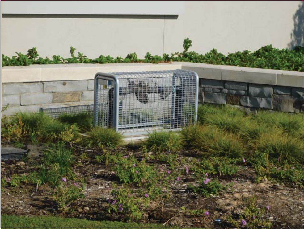
Drainage & Irrigation - Backflow preventer
