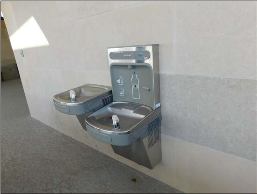
HVAC & Plumbing - Drinking fountain
