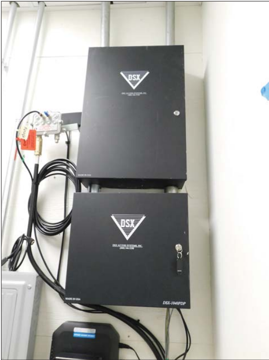
Appliances & Electronics - Access controller
