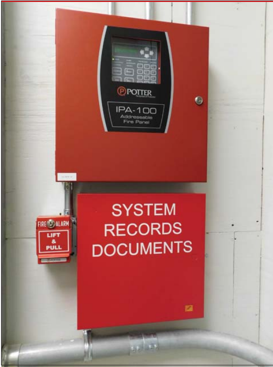
Appliances & Electronics - Fire alarm panel
