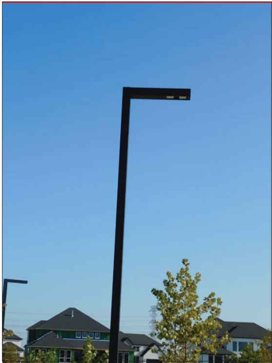
Lighting - Typical pole-mounted fixture
