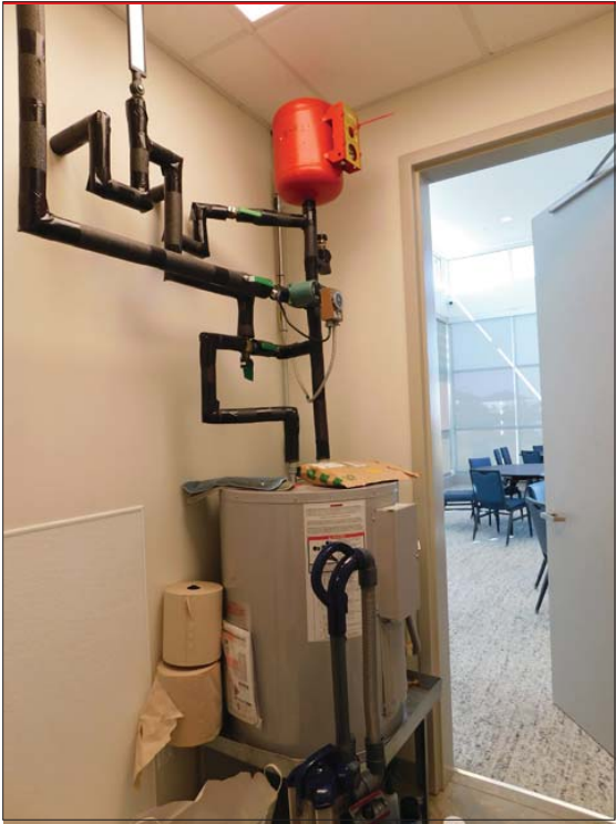
HVAC & Plumbing - Water heater
