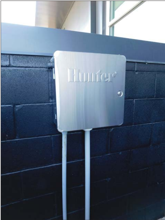
Drainage & Irrigation - Irrigation controller
