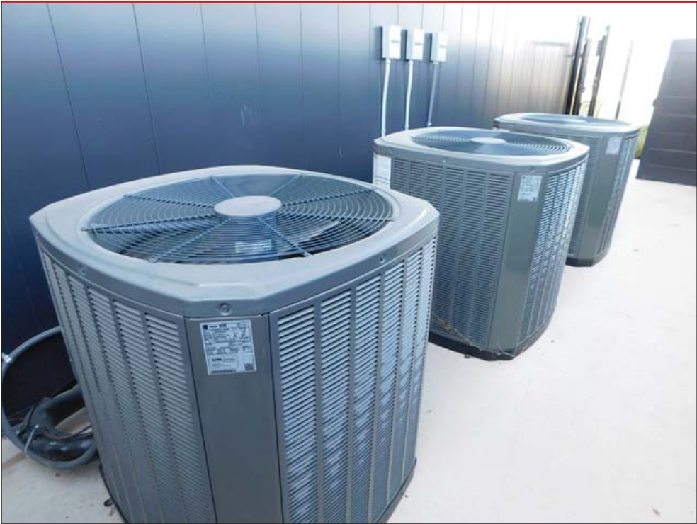
HVAC & Plumbing - Air-conditioners
